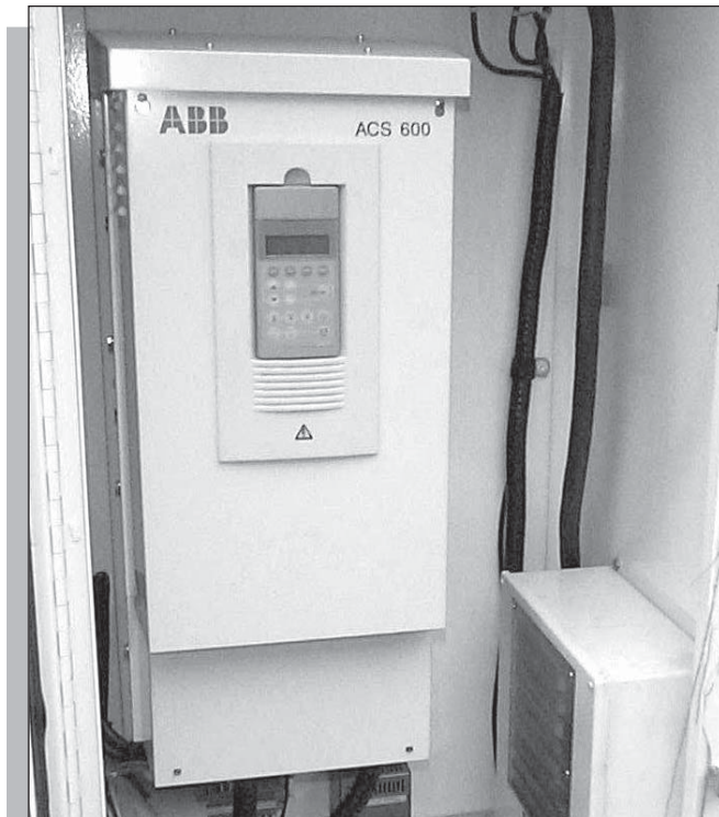
This variable frequency drive controller, which controls the speed of the motor driving the winch, is a compact unit that fits in an all-weather housing.
